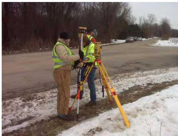
Gordon Warner, Civil Technician, is operating the robotic total station – an essential tool for designing and constructing infrastructure projects.
