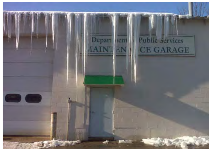
The Maintenance Garage is extremely energy inefficient, as evidenced by the extensive ice cycles. Weatherization is needed to save on energy costs.
